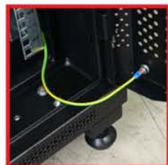
Grounding Connecting Between all Removable Part of Rack
